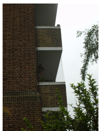
An example of netting used to protect a balcony.
